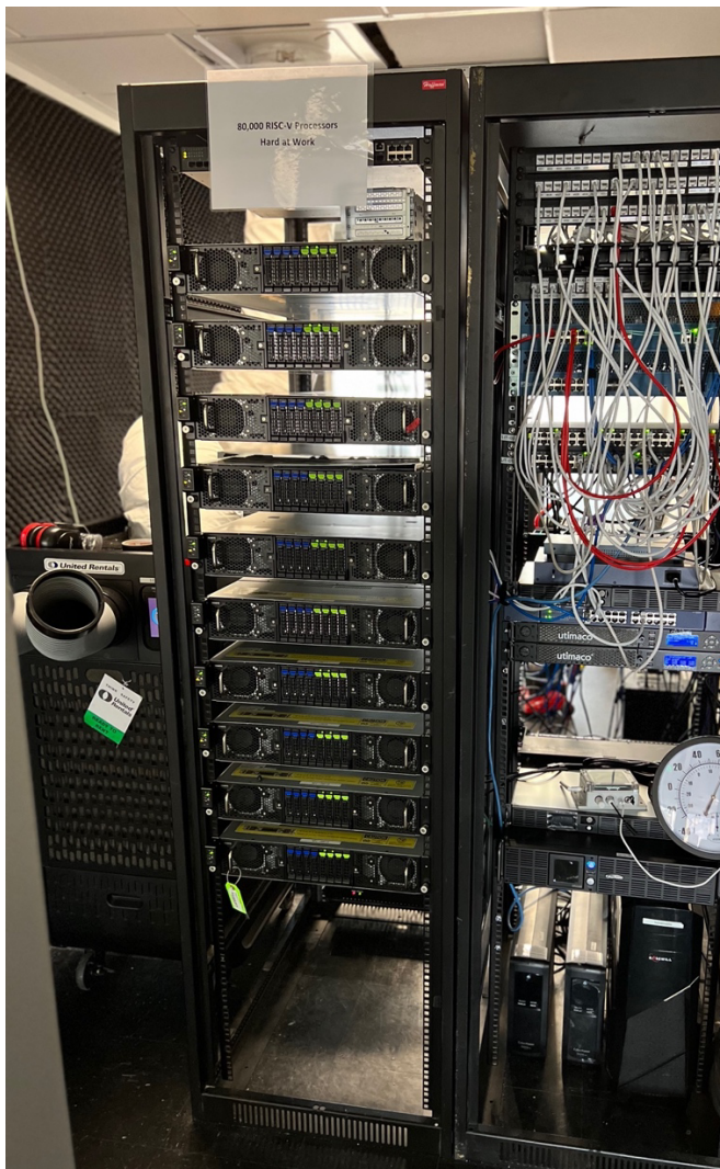
Figure 1. Example of Ten 2U Esperanto Servers with 87K RISC-V processors in this rack.
